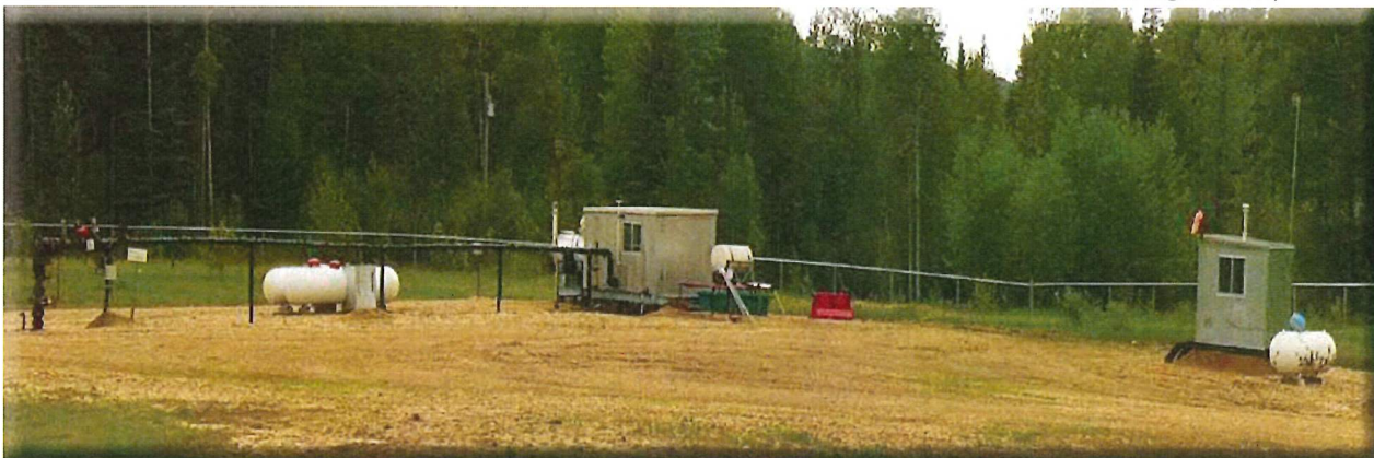
Natural gas facility
